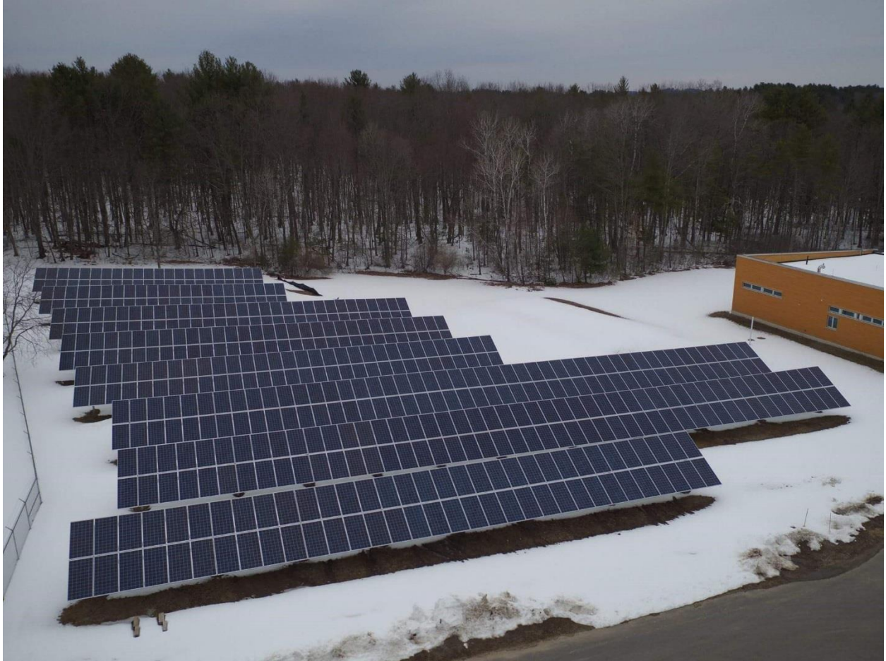
Madbury Water Treatment Plant
