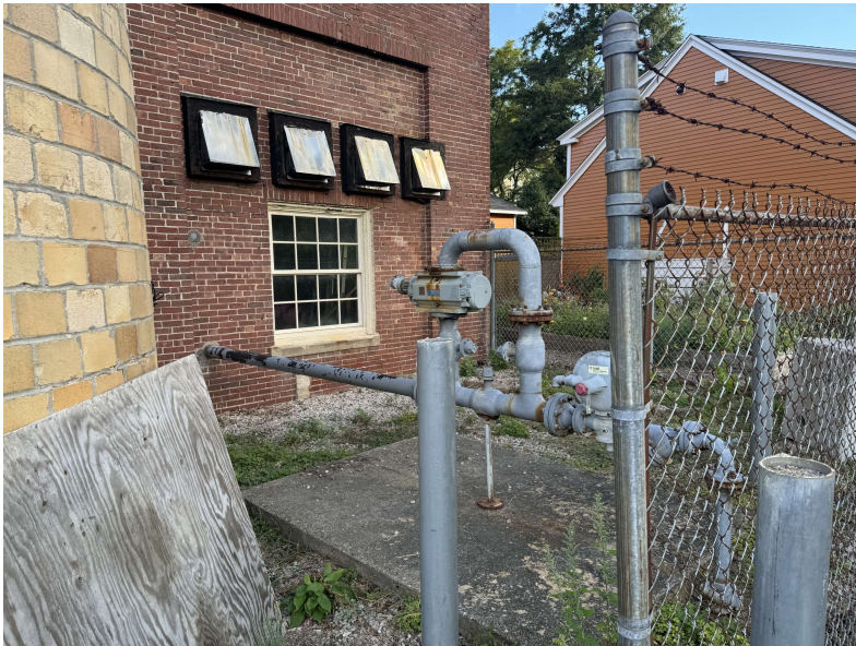
2013-2014 boiler system with Natural Gas
